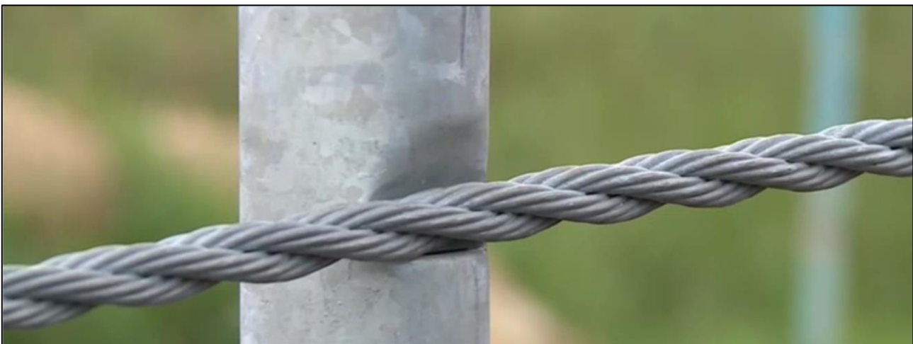
Figure 7: Rope Located within Recess of Line Post before Attachment of Retainer Clip
