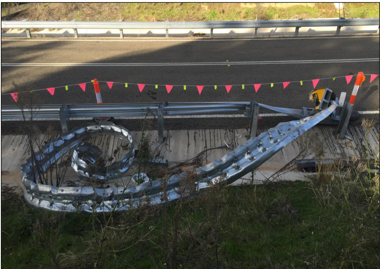
Damaged Rail after Travelling through Impact Head
